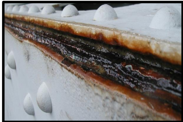
Figure 6. Crevice Corrosion Source: Orapi Asia, 2024
