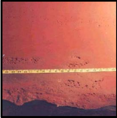
Figure 3. Pipeline damage from pitting Source: Pipeline and Hazardous Materials Safety Administration, 2019
