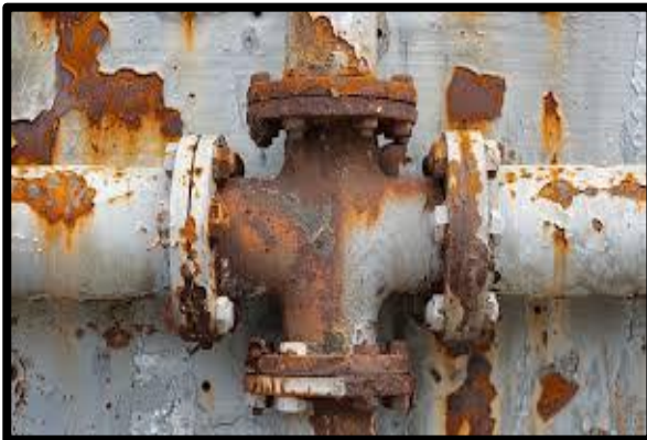
Figure 5. Galvanic corrosion Source: Galvanic Corrosion: Causes, Prevention and Testing. (n.d.)
